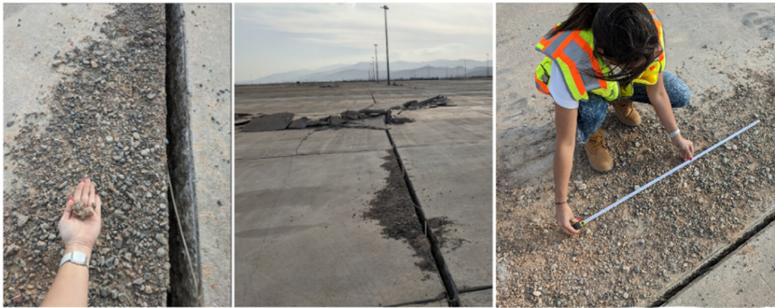
Figure 16. Observations of ground cracks and gravelly ejecta in the Lojistik area South of Türkoğlu (37.372 N, 36.861 E).
