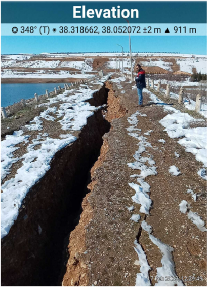
Figure 27. Crest cracking of the Sultansuyu dam (38.318662 N, 38.052072 E).
